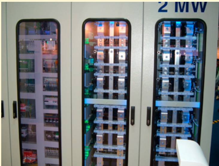
Protection of semiconductors inside middle voltage inverters.
